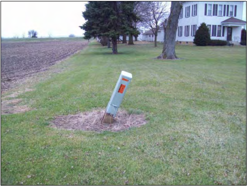
STANDING AT THE EXISTING TELCO PEDESTAL APPROXIMATELY 400' WEST OF THE SITE (LOOKING NORTH)
